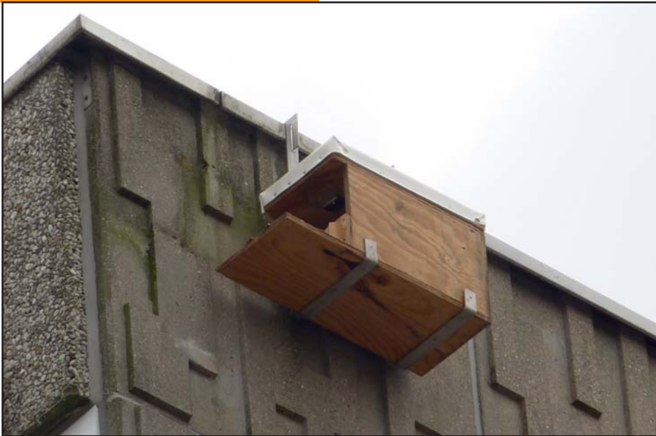
Kestrels have again moved into this nesting box.
